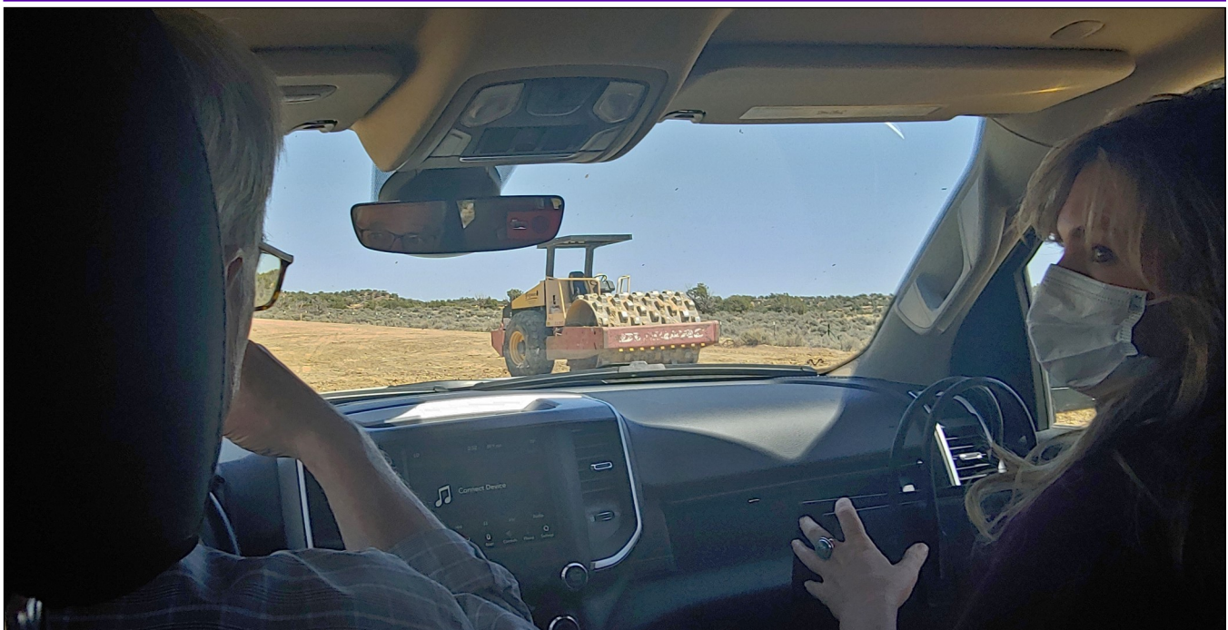
Martin O'Malley, General Manager of Gallup Land Partners & NMEDD Secretary Alicia Keyes survey Carbon Coal Rd. construction
